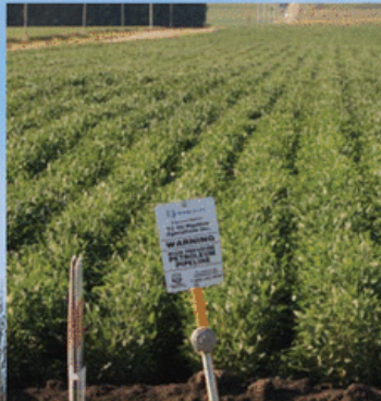
The Keystone right-of-way (above) near David City, Nebraska, demonstrates our respect for the land and the environment. We are committed to ensuring that any land disturbed by pipeline construction is fully restored.
